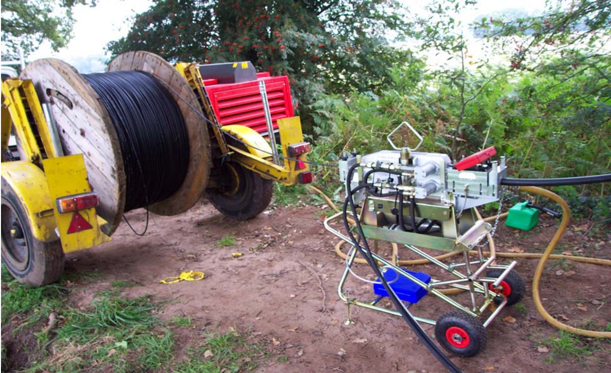
Figure 3: The optical fibre cable (stored on the reel) is 'blown in' to the duct (at right) using high pressure compressed air. This technique minimizes the risk of damage to the cable, both from snagging and by distributing the tension over the length of the cable
