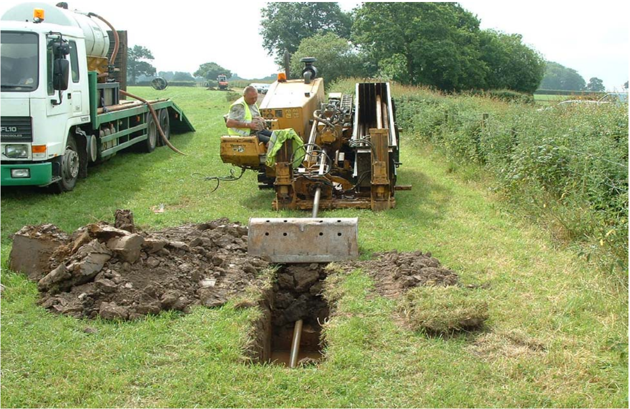
Figure 2: The horizontal directional drilling machine in action near the Pickmere telescope. This machine installs the cable duct at a typical depth of 1-2m in lengths of up to 100m. The depth and direction of the drill head is sensed and controlled remotely. This technique has allowed installation of the cable duct across farmland, underneath major roads and underneath driveways with minimal disruption.
